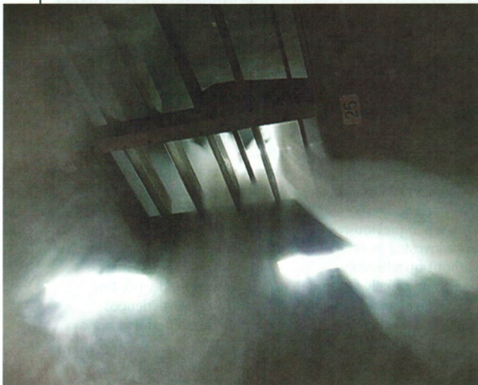
Below: Smoke exhaust damper in action
