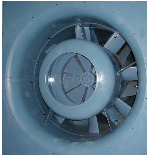
Figure 8: Pitot tubes in a fan inlet bellmouth for flow measurement
