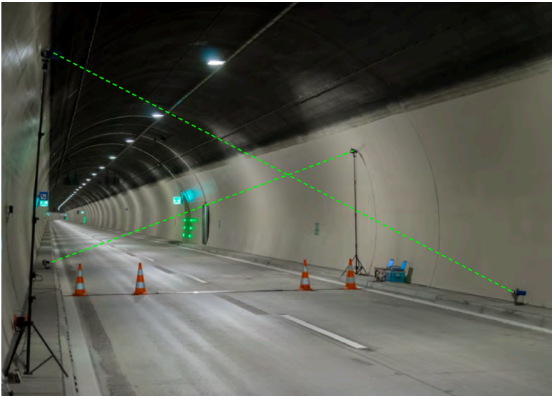
Figure 13: Cross alignment of ultrasonic line anemometers in a road tunnel
