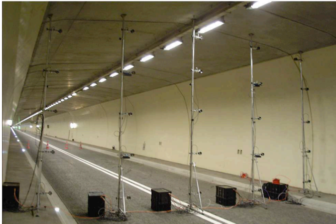
Figure 7: Flow measuring grid in road tunnel
