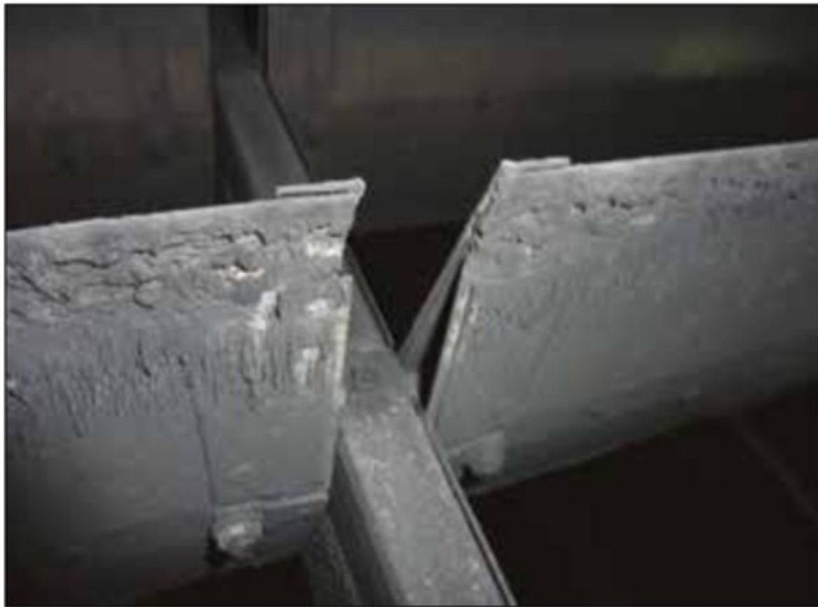
Figure 4: Exhaust damper blades in the Gotthard Road Tunnel after 10 years of operation
